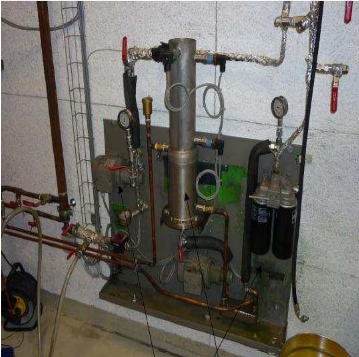
* Picture 9: Fuel transport unit with fuel pump, preheating (copper pipes for hot water supply) and fuel filters.
